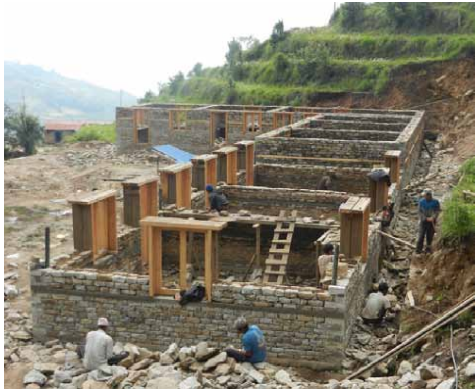
Construction of the Chhiringkharka Primary School in the Solukhumbu District of Nepal. Once completed eighty children from the village will be enrolled.
